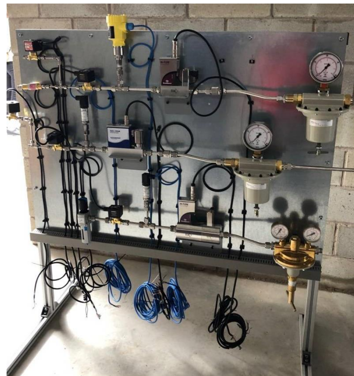
Panel de control
